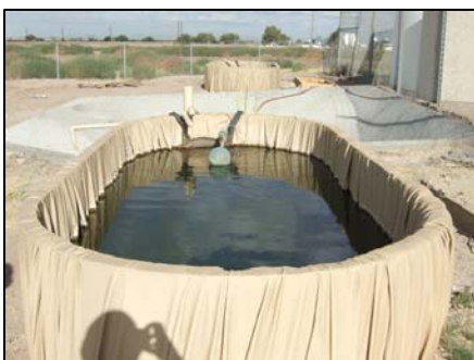
Slowsand filter after being filled up
