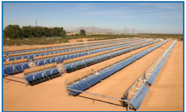
APS Saguaro Solar Facility, Red Rock, Arizona. Solar thermal plants like this one use water for cooling and mirror washing.
